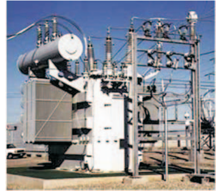
Figure 1.10 View of a Transformer
